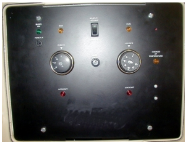
Control Panel up to October 2006
