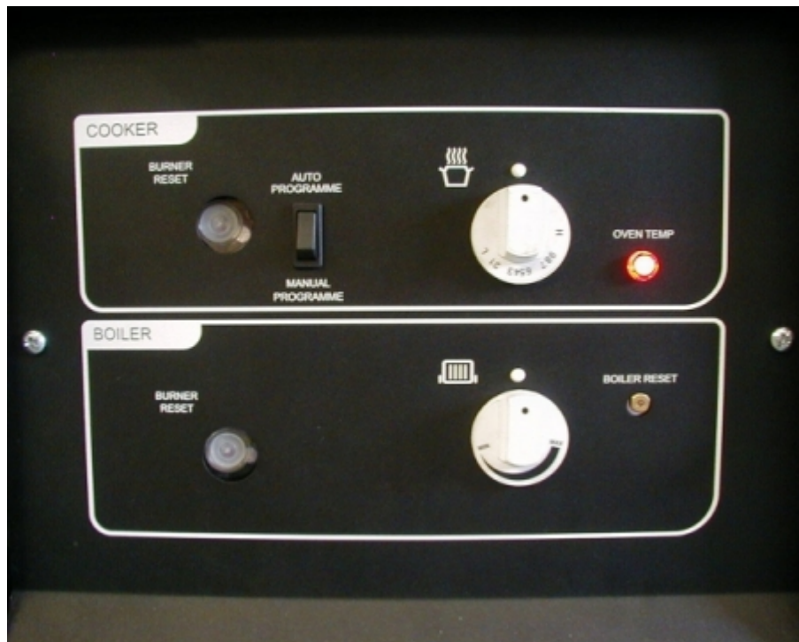
Current Control Panel.
