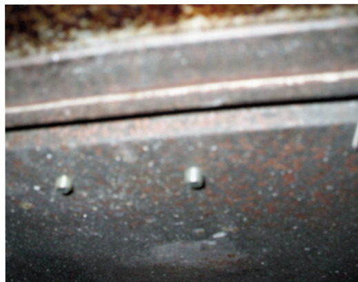
FIG. 6 STUDS PROTRUDING THROUGH ROOF OF OVEN
