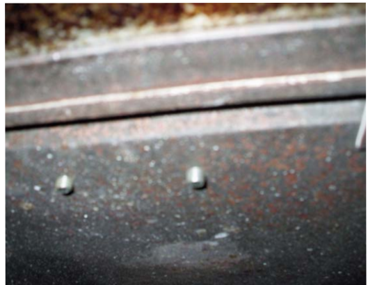
FIG. 6 STUDS PROTRUDING THROUGH ROOF OF OVEN
