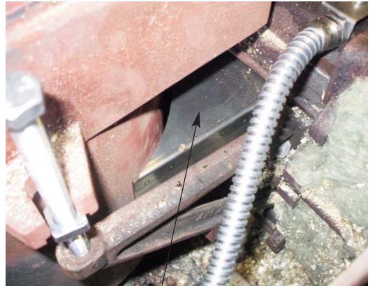
FIG. 4 FIT TUNNEL BETWEEN BARREL & OVEN
