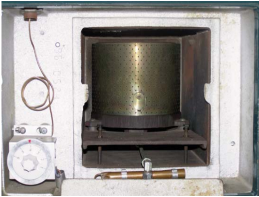
FIG. 1 OIL CONTROLS TO BE REMOVED
